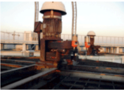
• Motor Bearing in Cooling Tower (Amusement Park)
